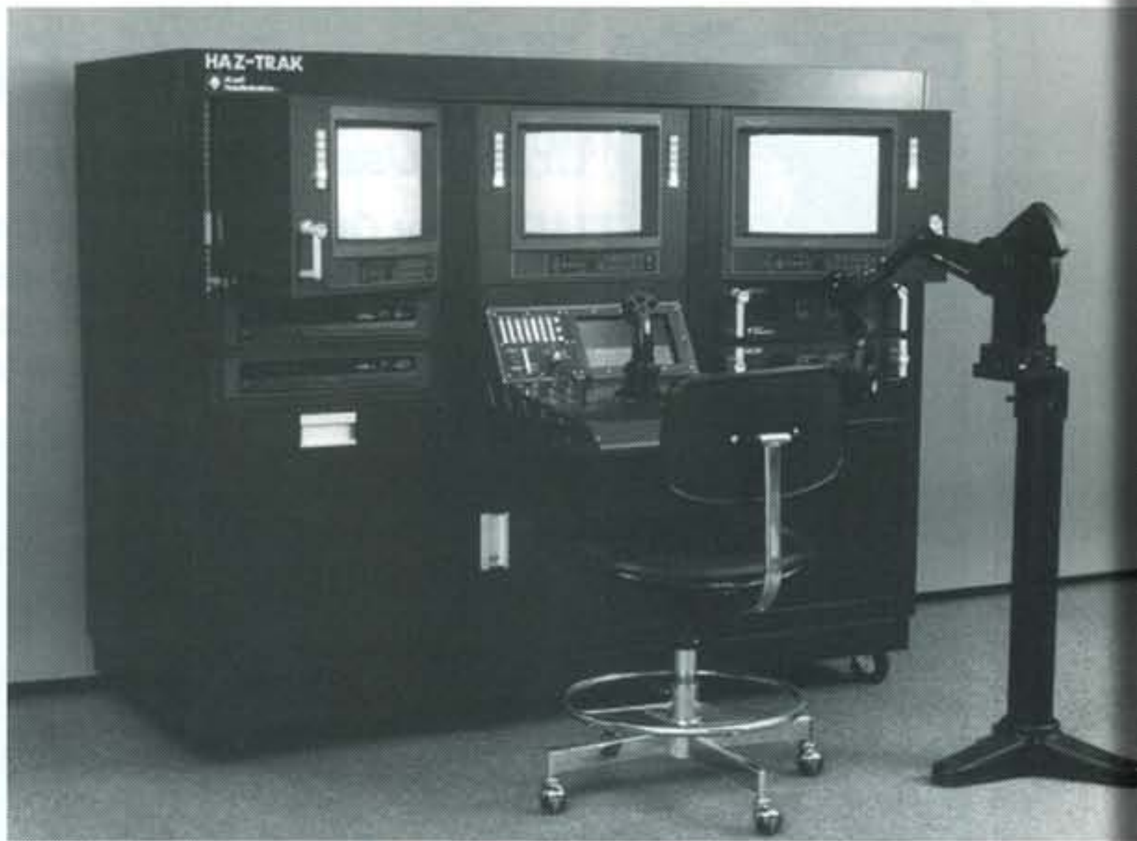
The control console is designed to permit full system operation by a single person from the center bay.
