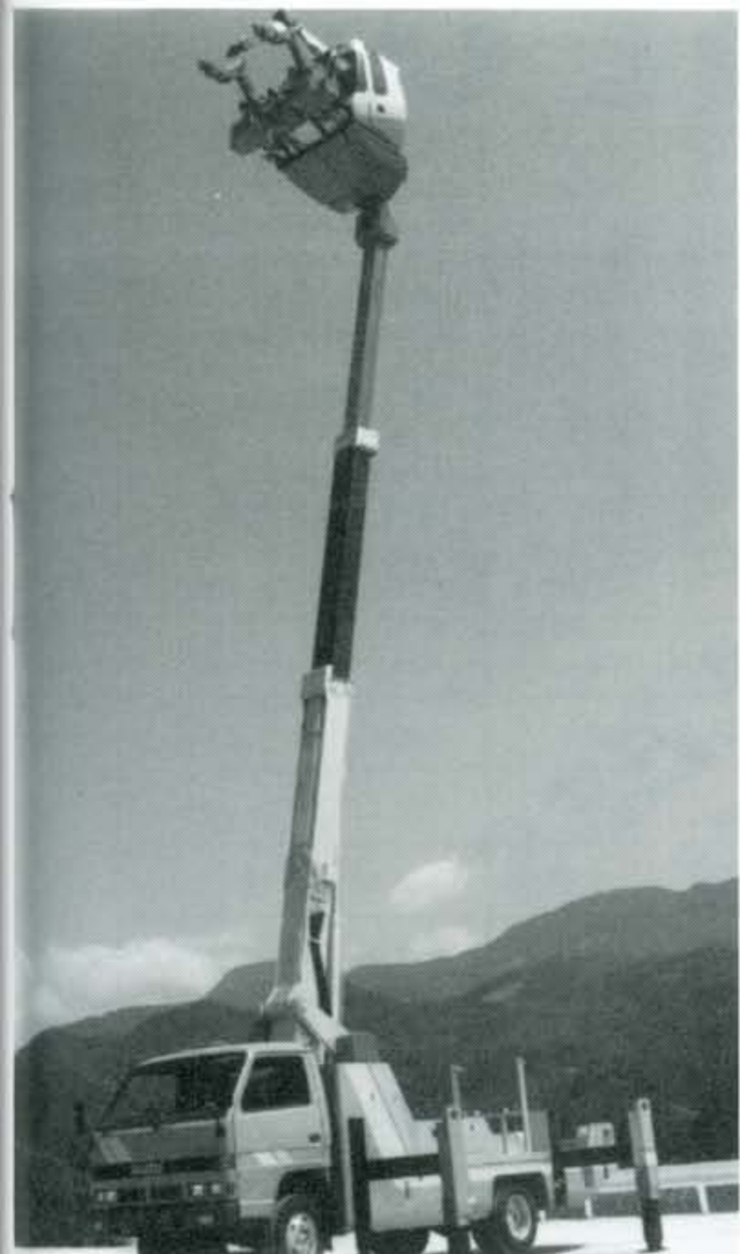
A lineman operator using two insulated force feedback manipulator arms, is ready to perform a variety of complex tasks on energized distribution lines.
